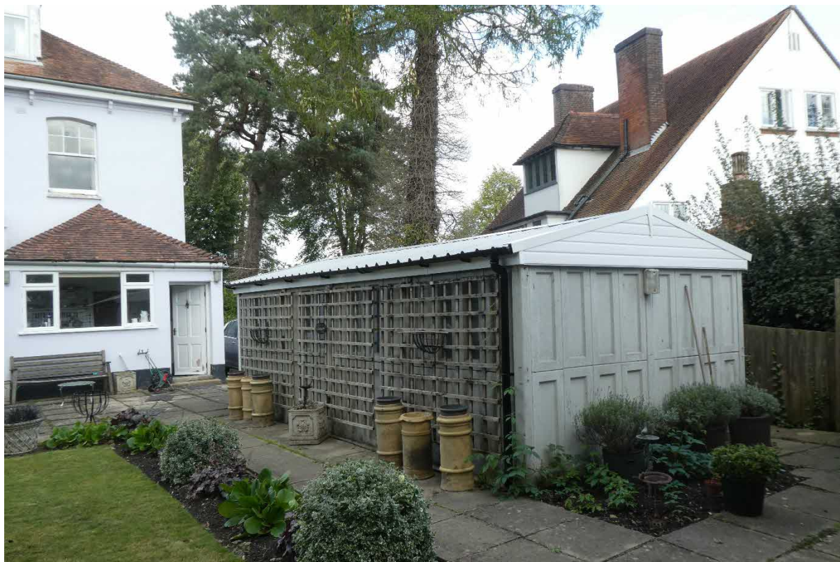
127 Hadham Road, CM23 2QD: photographs taken after work on garage roof completed
