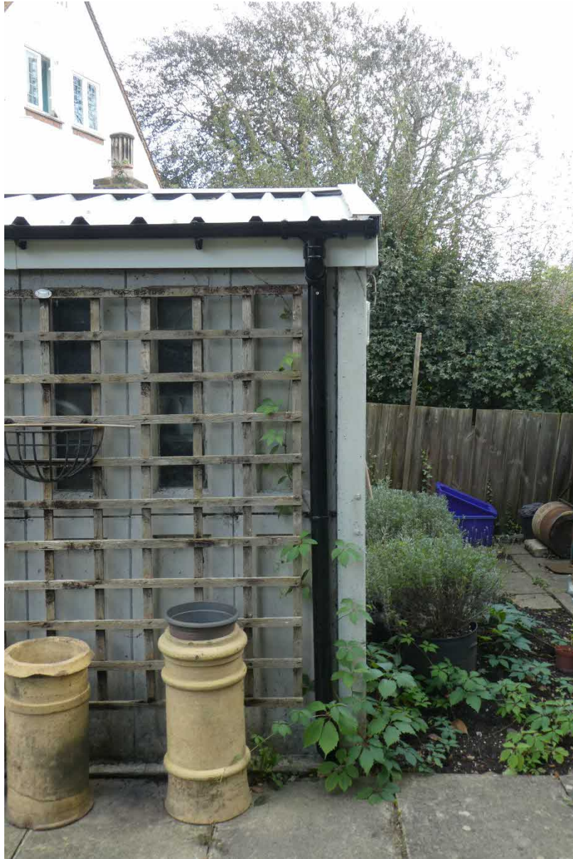
127 Hadham Road, CM23 2QD: photographs taken after work on garage roof completed
