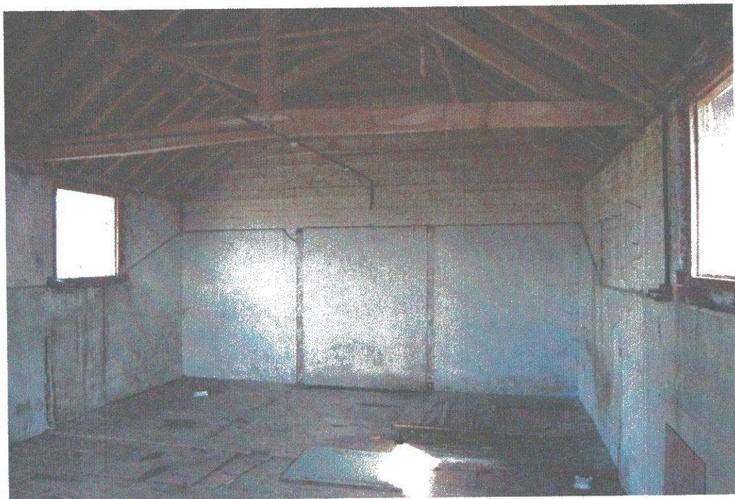
Plate 12: South outbuilding interior showing evidence of former grain bins and the crown post roof structure.
