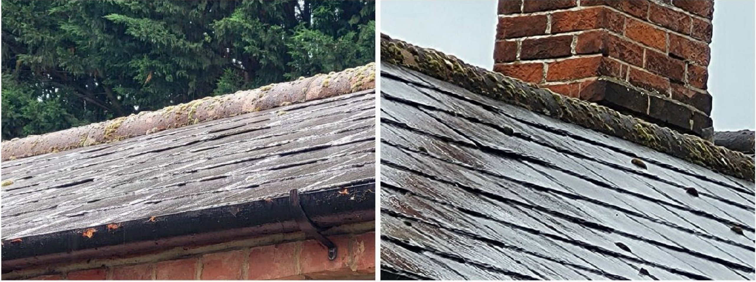
Figure 7. Example of slightly lifted roof slates
