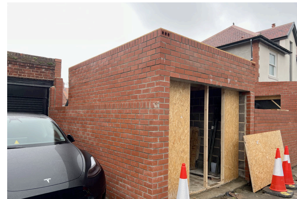
fig 7: Photo taken on 11th March 2024 showing garden store and rebuilt garden wall to adjacent property. There will be painted timber inward opening doors fitted to the opening.
