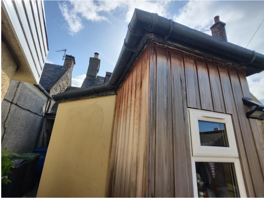
Timber clad rear porch- suggesting the use of timber as a unifying medium
