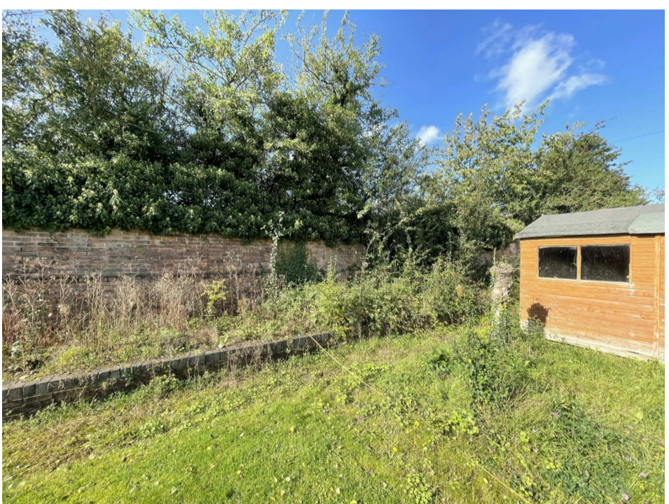
Photo 7 The 'Garden Walls' separating the 'side garden' from Blithbury Road. These are historic red brick walls which exhibit mixed brick bonding. There is some evidence of Flemish Bond, some evidence of 'English Bond / English Garden Wall Bond, some Stretcher Bond' all capped with a decorative brick coping.
