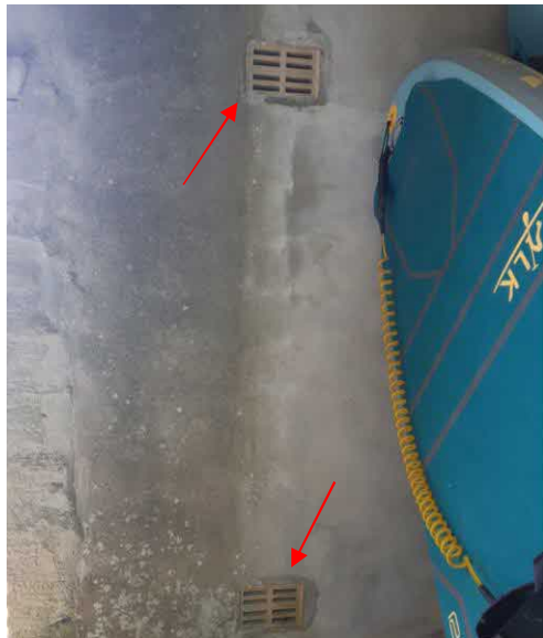
Figure 9. Vents in store building
