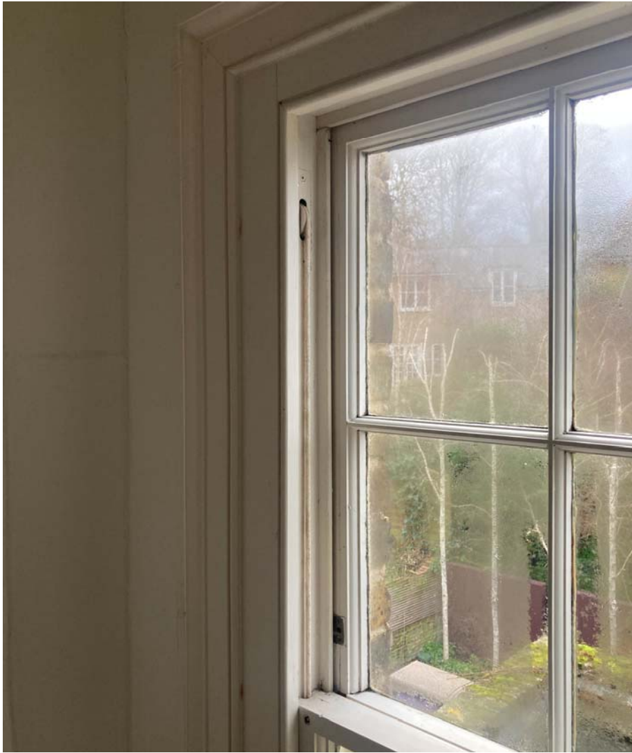
Photo 18: Second floor landing window condition
