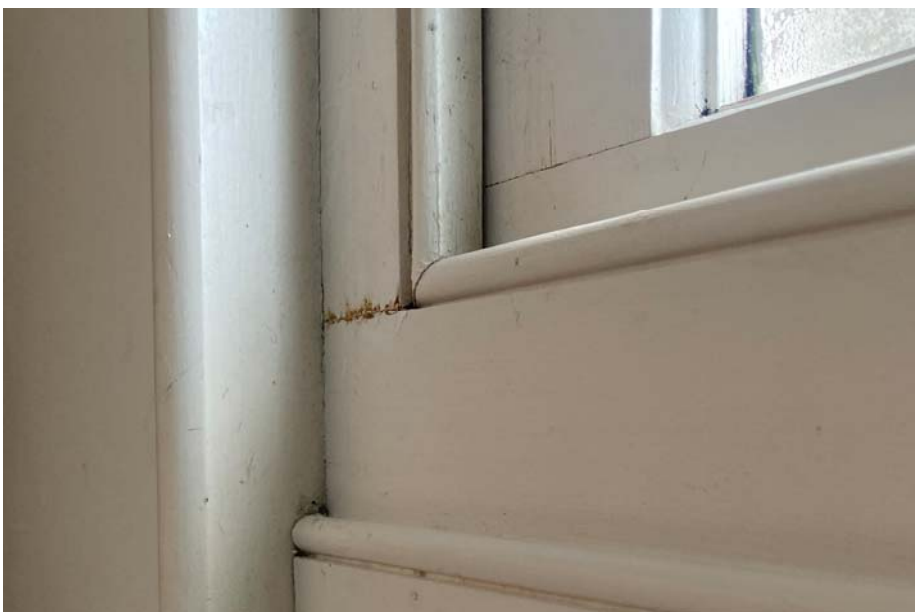
Photo 19: Second floor landing window condition
