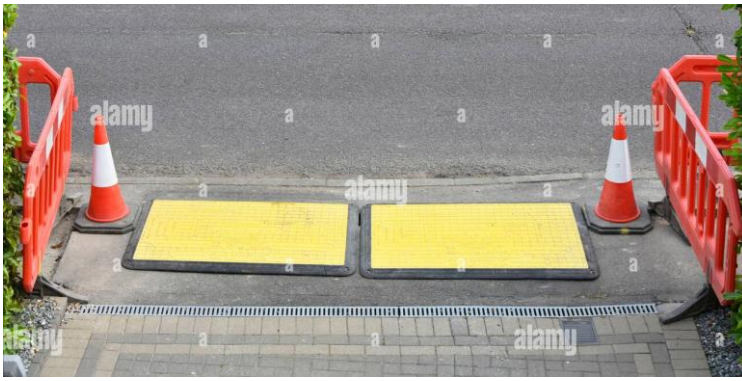
Figure 11.a: An example of the temporary HDC set up along the main access points on the footway during the construction period.
