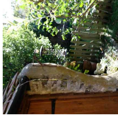
2.10 View of the end of the historic flint wall, that forms one side of the building.
