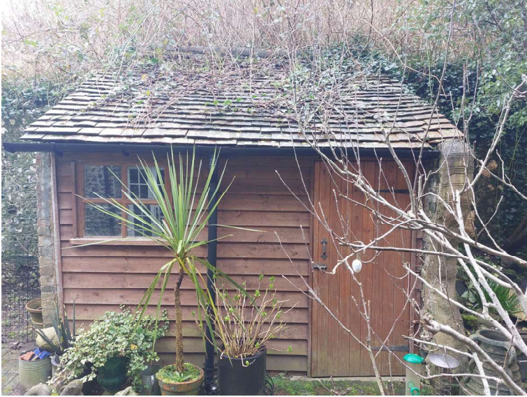
Image 03 – View of front of B01, showing uneven and raised tiles, and timber cladding front.
