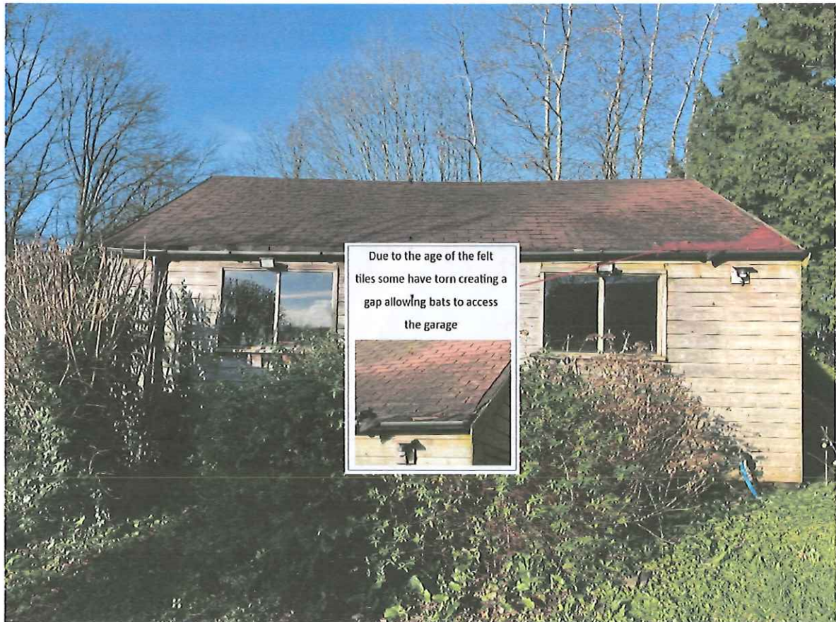
Image 4.3.1.1. Location of potential bat access point on the east elevation of the double garage.
