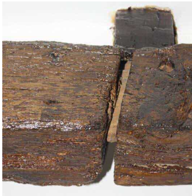
Plate 14. Crude lap-joint in the wallplate.
