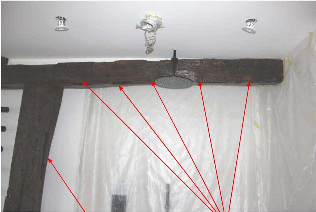
Plate 13. Empty mortice for missing foot brace and close studding mortices.
