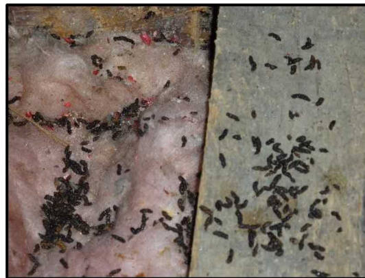
Long-eared bat droppings in roof void
