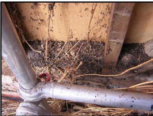
Pipistrelle droppings in exposed wall cavity
