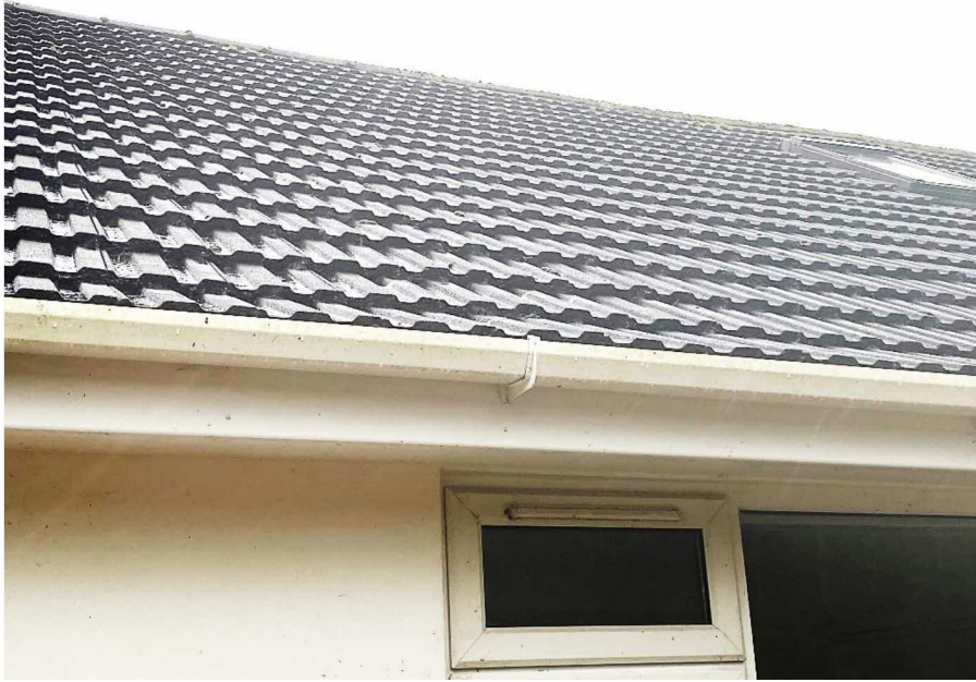
Tightly sealed eaves and roof tiles at the front (north) side of roof
