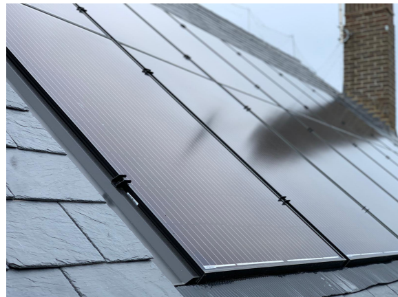
3.8kWp Photovoltaic Array
