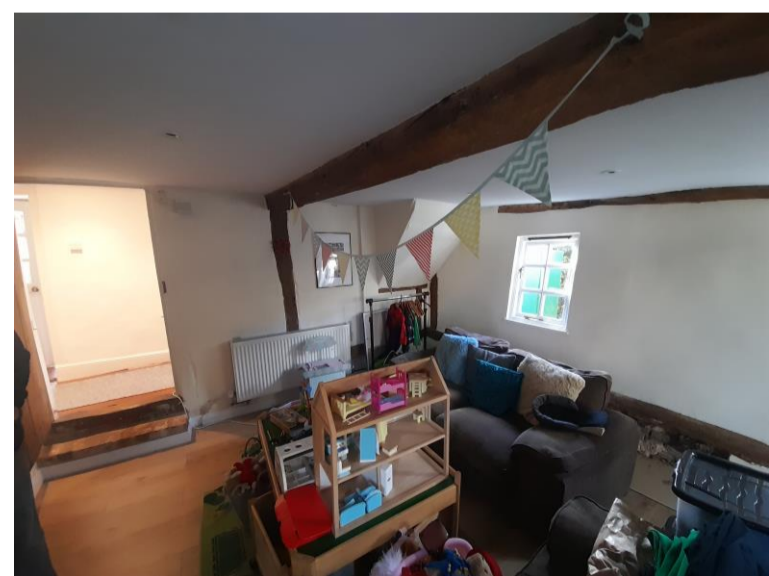
Image 11 View to left of brick pier showing historic beam (to be retained)
