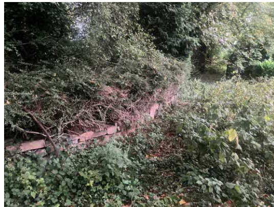
Photographs 3 – The small retaining wall at the front (north of the site) where trees are growing along the northern boundary. A section will need to be removed for the proposed access road.
