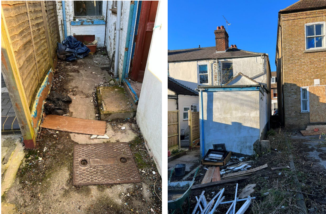
Figure 11 - Existing manhole cover at rear of property determining depth of new extension.
