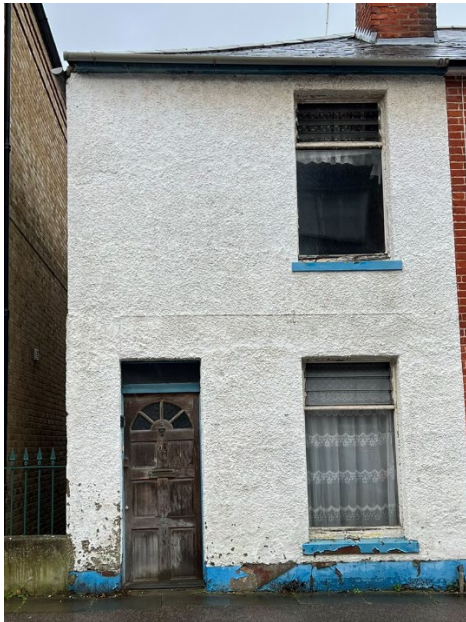
Figure 7 - Photo of no. 53 in current poor condition.
