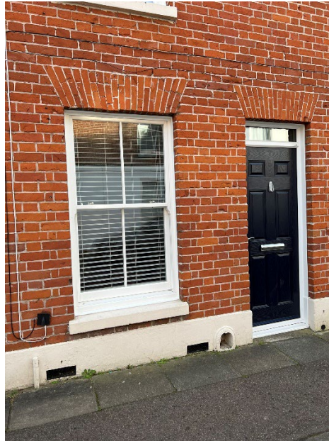
Figure 8 - Photo of no.55, exposed red brick, wood-effect uPVC sash window and black composite door.
