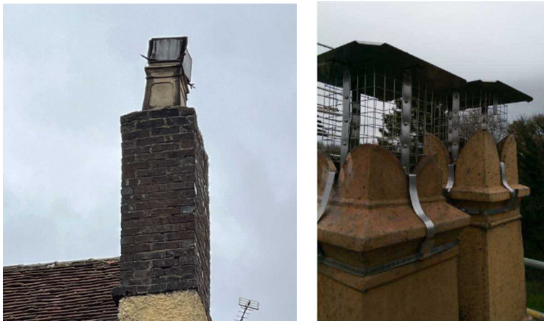
Figure 5: left - existing chimney, right - proposed stainless steel cowl to go on chimney.
