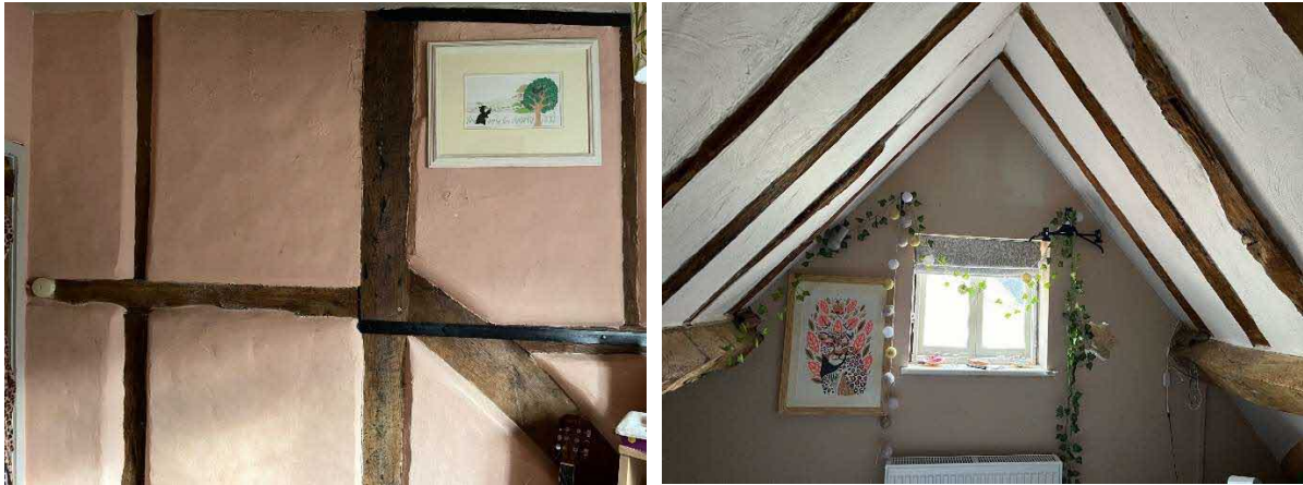
Figure 4: Left – exposed timber in the first floor bedroom indicate the condition of the timber beams is good. Right – attic room where the timber frame to the north east gable is concealed by internal finishes
