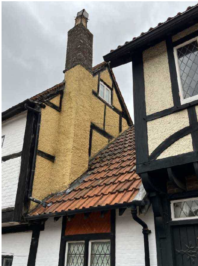
Figure 3: rough cast concrete and mock tudor beams concealing timber frame and brick infill panels.
