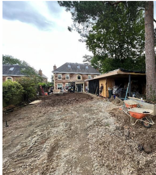
Re-use existing open grade Sub Base topped up to a minimum of 150mm Type 3 open grade hardcore
