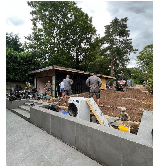
150mm Sub Base well compacted Type 3 open grade hardcore with reduced fines.
