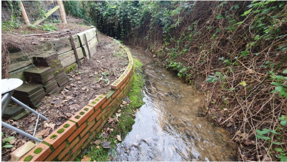
Photograph 3. Watercourse adjacent to the Site, showing brick reinforcement of the bank toe and further timber reinforcement higher up the bank.
