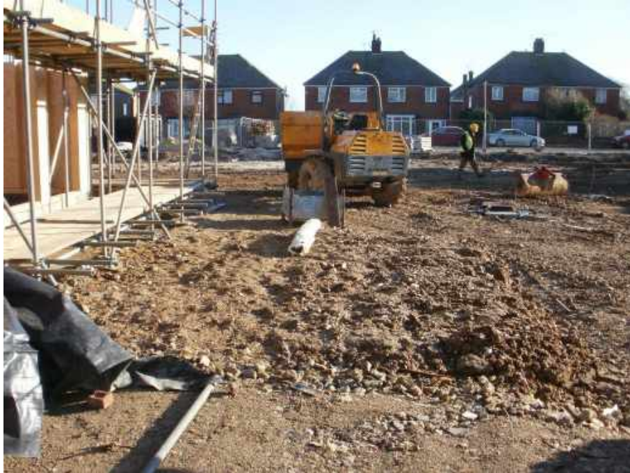
Looking east across the centre of the southeast area of the site showing the natural ground (head deposits) at the location of the proposed gardens to plots 12 to 14.
