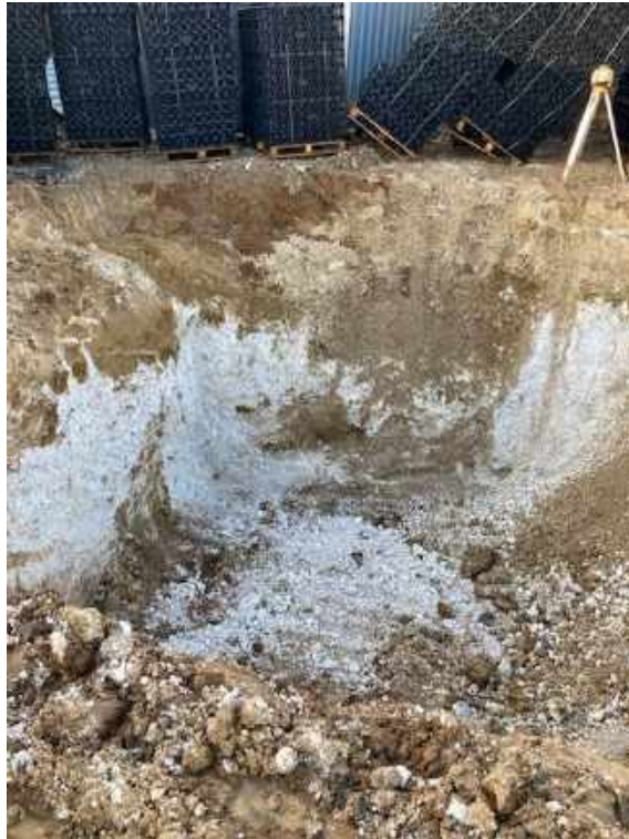
Excavation of the soakaway in the southwest area of the site showing the expected natural ground.
