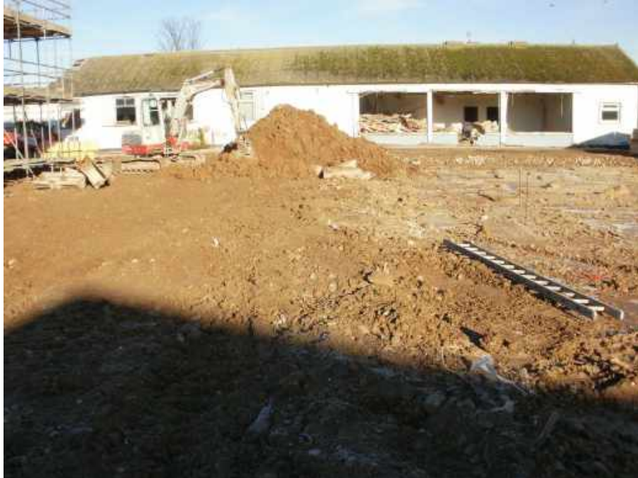
Looking north across the southeast area of the site showing the natural ground (head deposits) at the location of the proposed gardens to plots 15 to 23. A small public open space area for the planting of a small tree will be in the background on the right.
