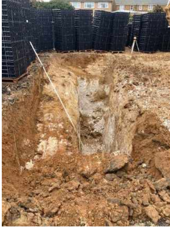
Excavation of the soakaway in the southwest area of the site showing the expected natural ground.
