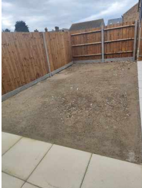
One of the plots with the sub base laid for the artificial grass.
