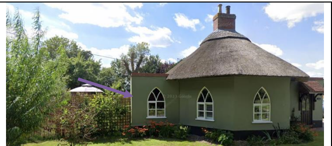
Extension to be added onto the south-eastern elevation (onto lawn). Flat roofed area will be replaced with a pitched roof and cut into thatch.
