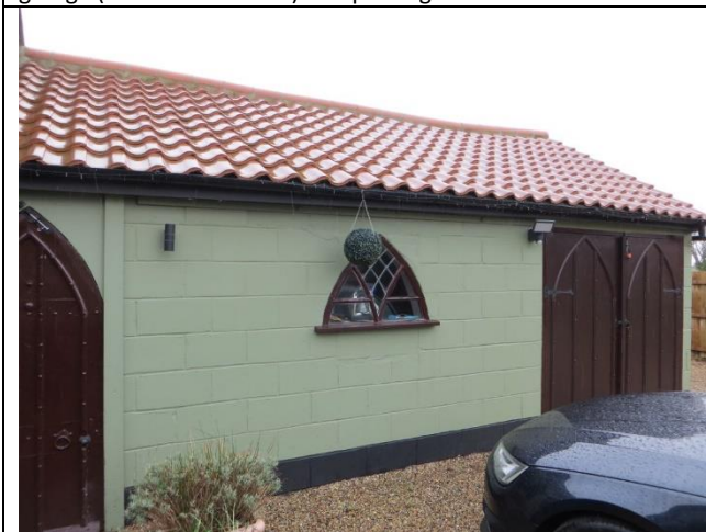
Existing garage. Re-roofed in the last two years. No gaps under tiles. All end tiles have plastic grilles to prevent ingress of mammals.
