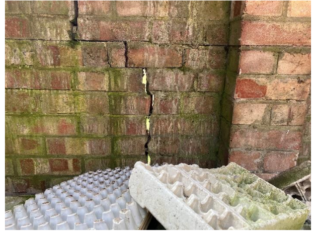
Photo 6: Typical crack in single skinned brickwork, running from inside to outside with no other cavity access
