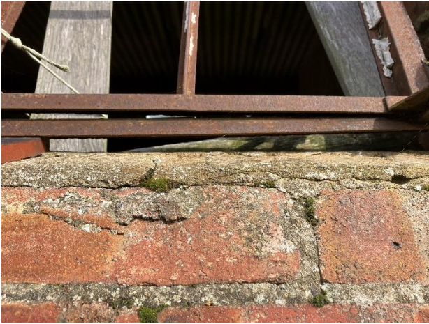
Photo 5: Gap between metal window frame and brick wall due to missing windowsill tiles
