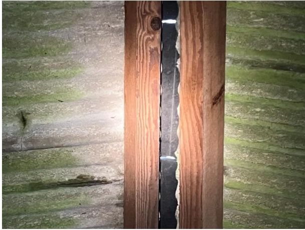
Photo 11: Large void at ridge between ridge tiles and adjacent beams
