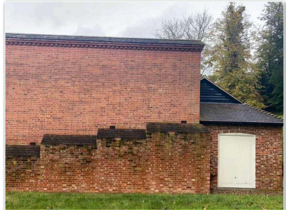
Brick Wall with Parapet to Nether Hall, a more recent addition to the original house.
