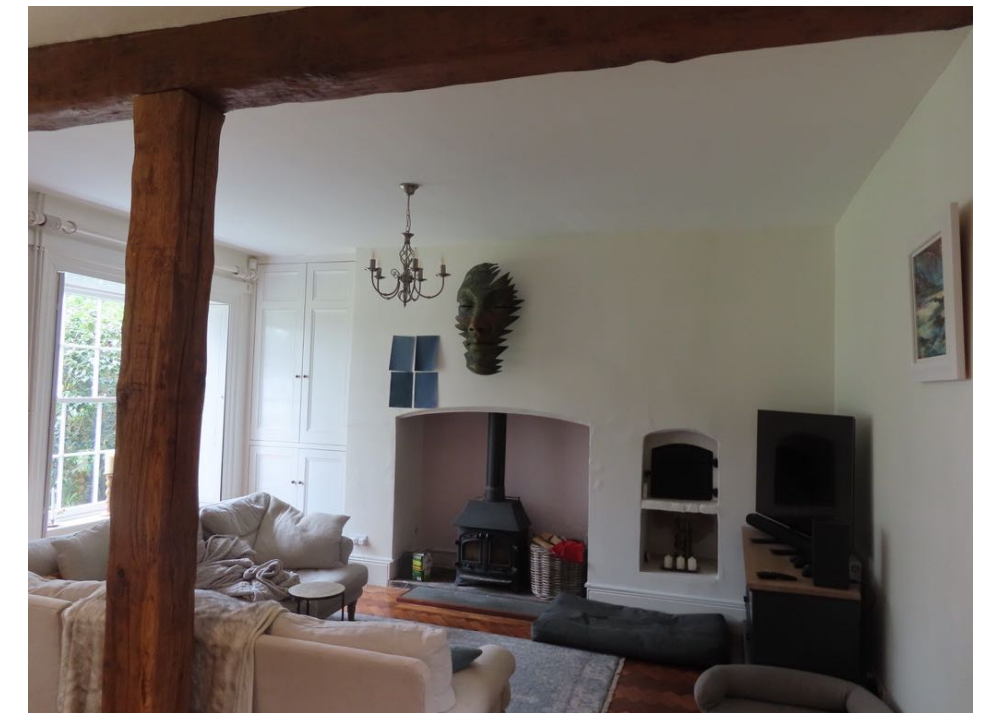
View of the north side wall with inset fireplace and bread oven part of the oldest area of the welling. This suffers from damp and will be remedied by hacking off the internal layers of modern plaster and using breathable lime plaster throughout.
