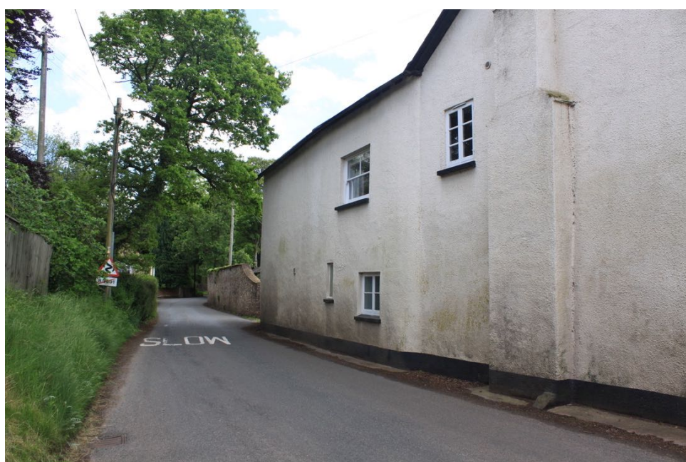
View from the public lane. The hard cement render will be replaced with a stone plinth at road level and lime render above at first floor.
