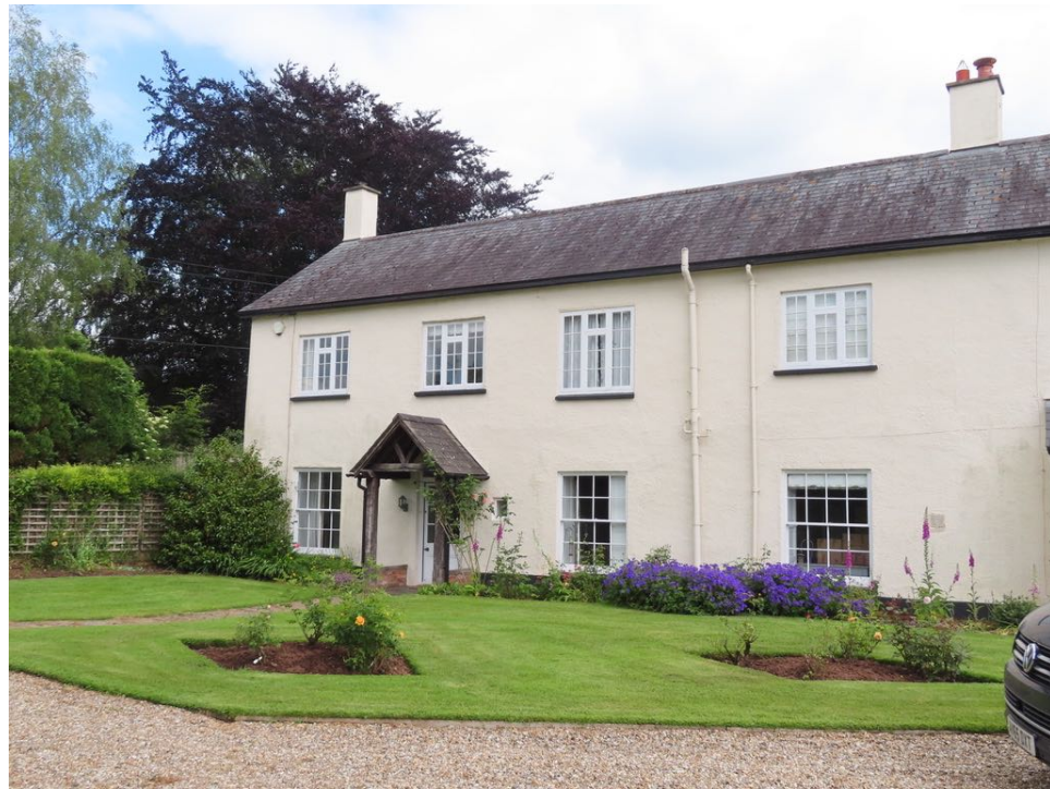
Photo of the western facing elevation with the principal entrance door in current location. The proposal is to replace the first floor casement windows with high quality traditional joinery flush casements.
