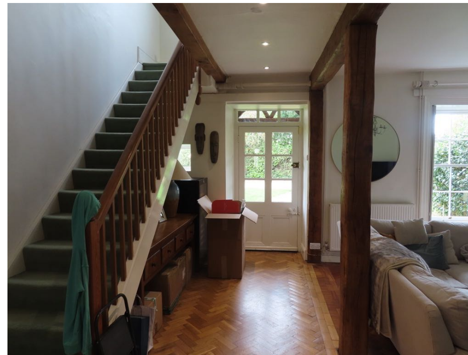
The secondary 20th C stair and opened up internal wall. The posts and beam are also 20th C infill and not wholly structural.
