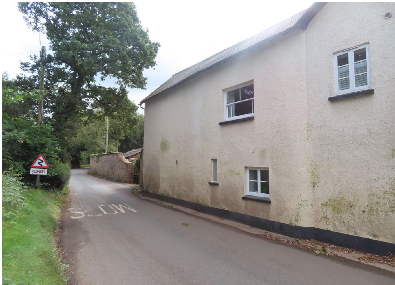
Northern facade addressing the public road. Significant internal damp caused by the hard cement render. This will be removed.
