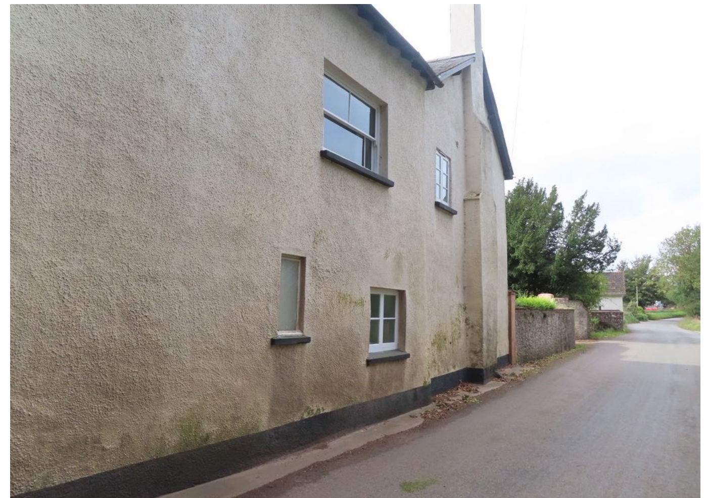
A new plinth of exposed stone will be formed as the existing stone wall to the house. Pointed with NHL 2.5 lime putty mortar and then fully lime rendered first floor above.
