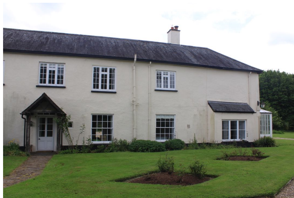
View of the west facing elevation. The first floor casement windows are relatively crude softwood painted type from the mid - late 20th Century.
