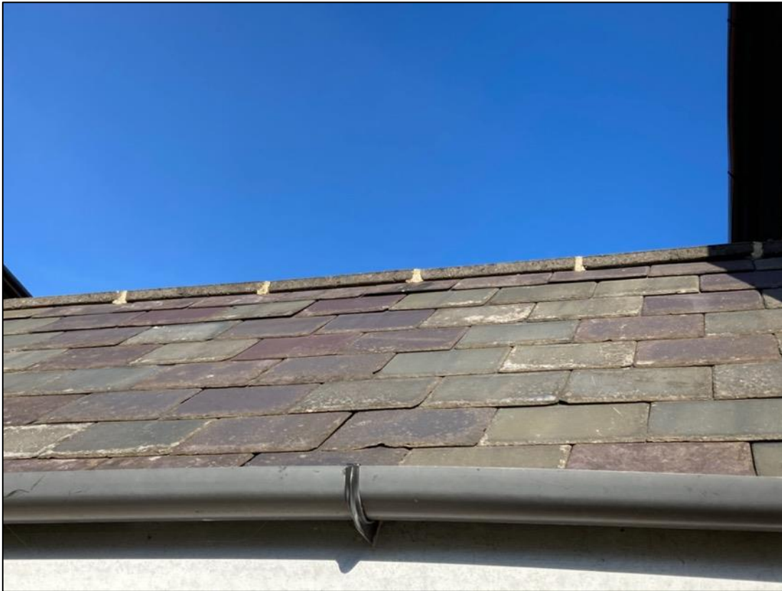
Photograph 3. Raised roof tiles and gap in ridge tile on southern aspect of house
