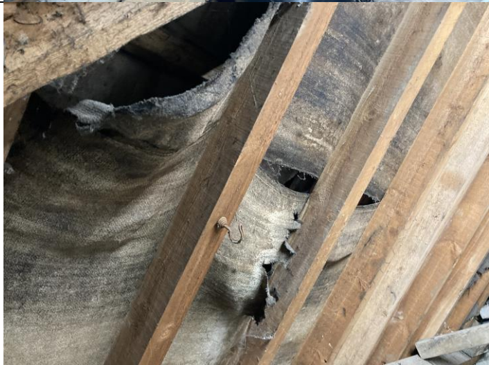
Photograph 3: Tear in the lining in the southern section of the roof void.
