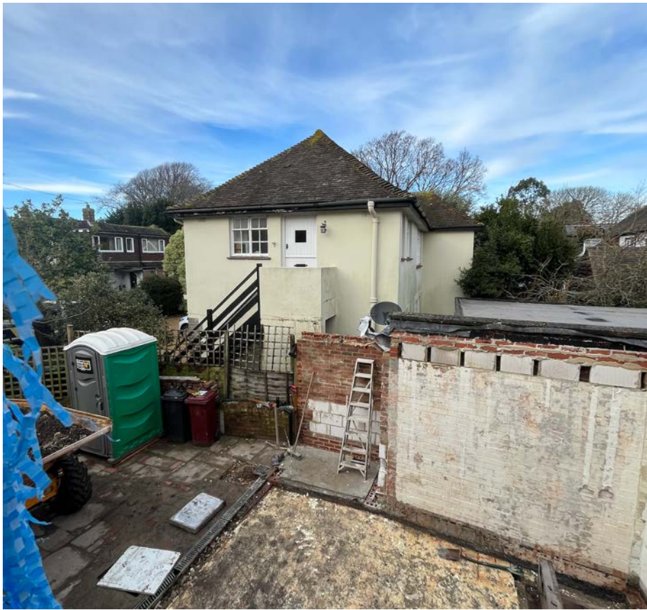
Figure 17: Photographs of the wall forming part of Somme Cottage that they hope to amalgamate with the new extension. The photographs have been taken following demolition of the rear extension that was previously attached to Corner Cottage (approved under 23/01237/DOM and Listed Building reference 23/01238/LBC)
