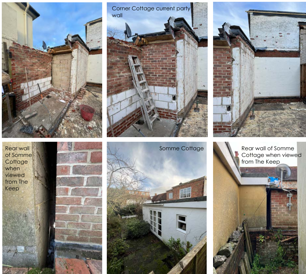
Figure 16: Photographs of the wall forming part of Somme Cottage that they hope to amalgamate with the new extension. The photographs have been taken following demolition of the rear extension that was previously attached to Corner Cottage (approved under 23/01237/DOM and Listed Building reference 23/01238/LBC)
