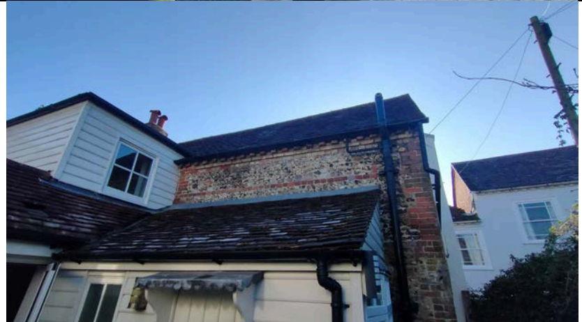
Photograph 3: Overview of the northern aspect of the building showing the lean-to to be demolished
