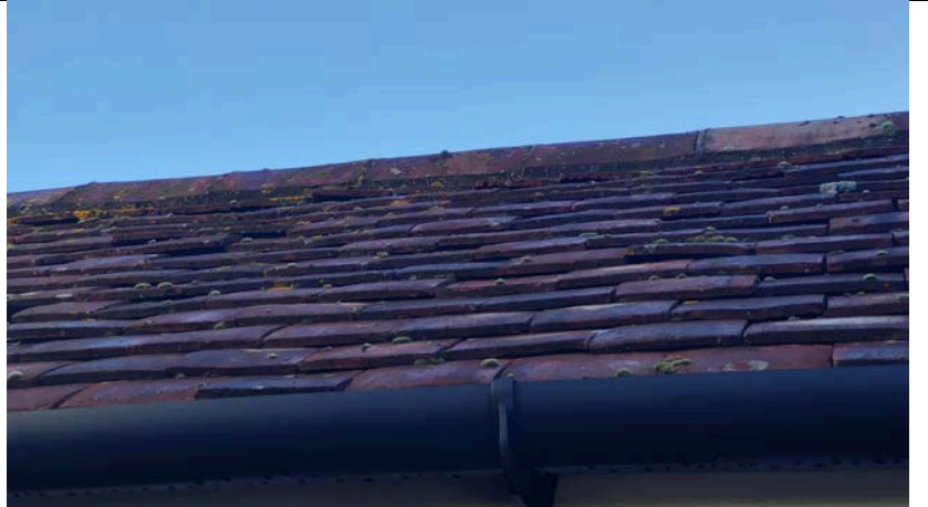
Photograph 5: Close-up of lifted tiles
