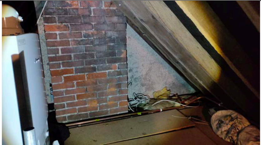
Photograph 1: Eastern end of the void in the older section of the house
