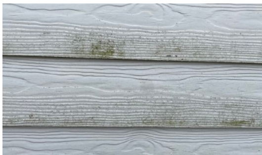
Existing weathered white cladding
