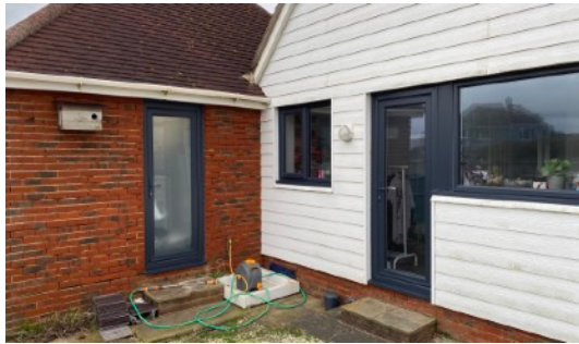
Inconsistent wall treatment
