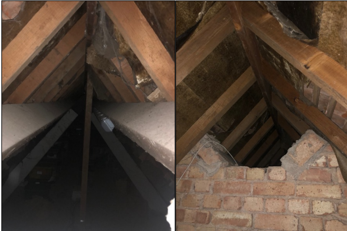
Photograph 4. (Left) Internal view of the larger loft void with torn bitumen lining the roof. (Right) The large gap between the two voids illustrating that for bats the two voids are interconnected.
