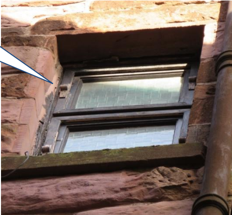
Zoom view showing style and deterioration
