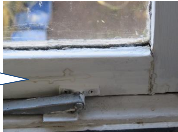
Internal view showing rot and leakage
