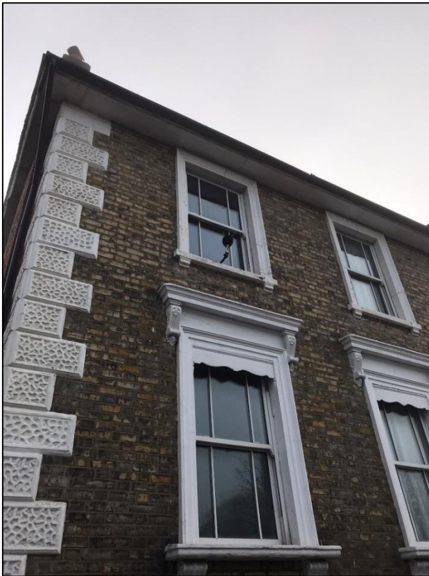
Figure 5 External facade showing the worst affected windows
