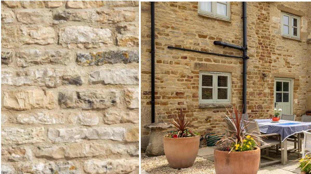
Typical random coursed stonework in lime mortar and “typical” wood casement windows.
