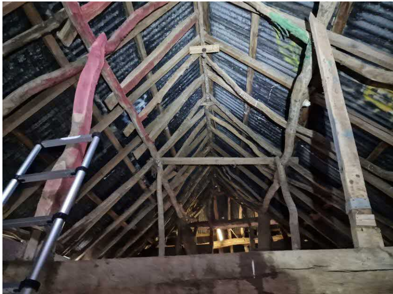
Photo 8: Internal view of the old stables showing the variety of old untreated wood used in the roof construction.
