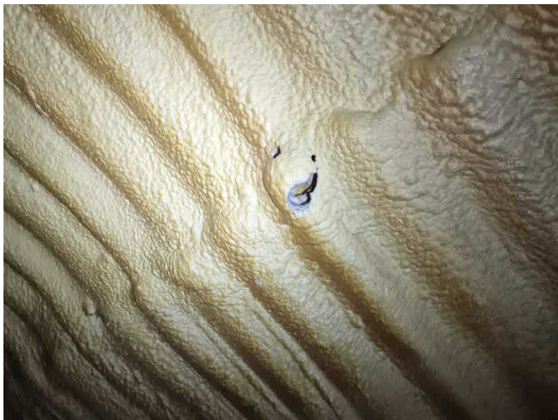
Photo 4: Internal break in the insulation having been used by nesting birds.
