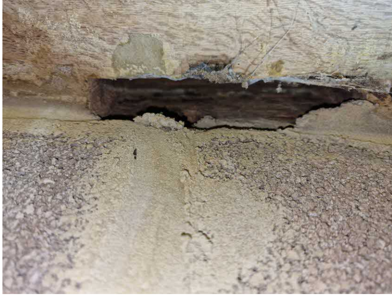
Photo 8: A gap between the brickwork and the roof timber with a bat faeces stuck to the wall.
