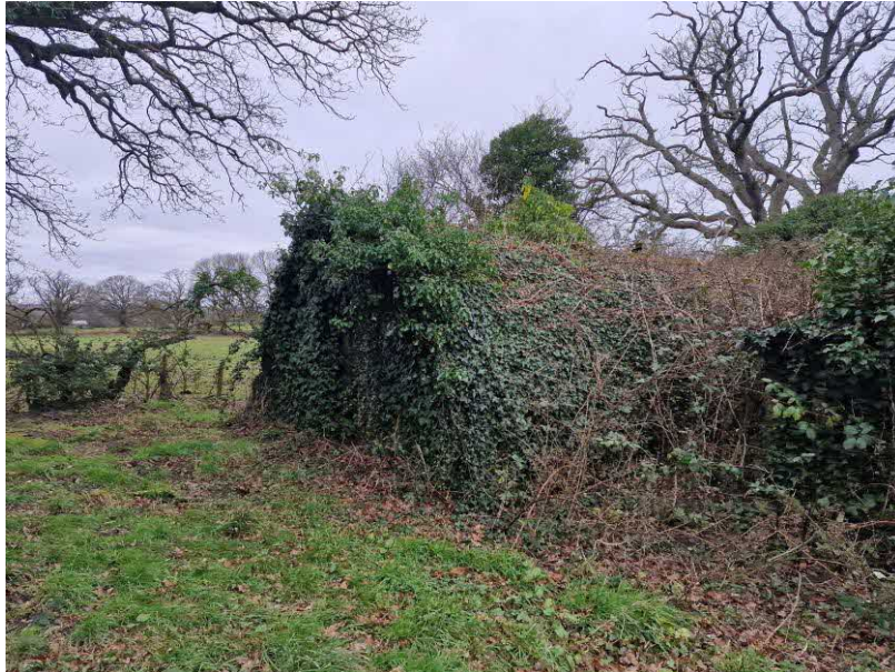
Photo 3: Corrugated metal shed covered in bramble and ivy.
