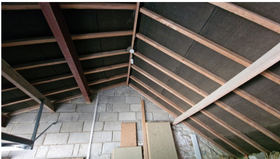
Image 4 - Interior showing C20th roof construction and purlin to be replaced with steel to right of image
