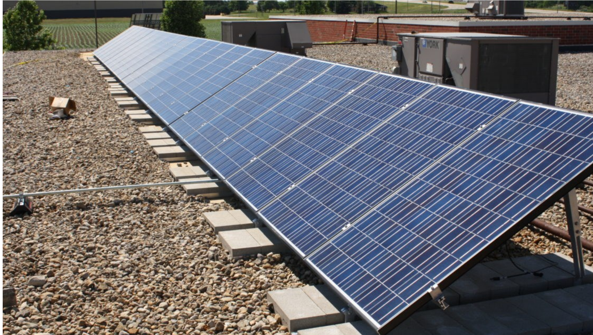
Fig 11.1 Ballasted Roof Mount Solar Panels
