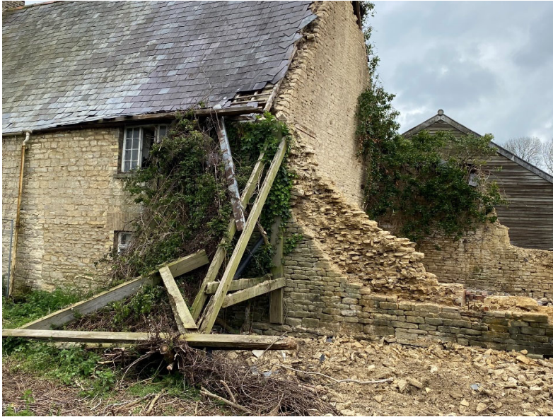
Cottage 2 rear elevation and collapsed barn
