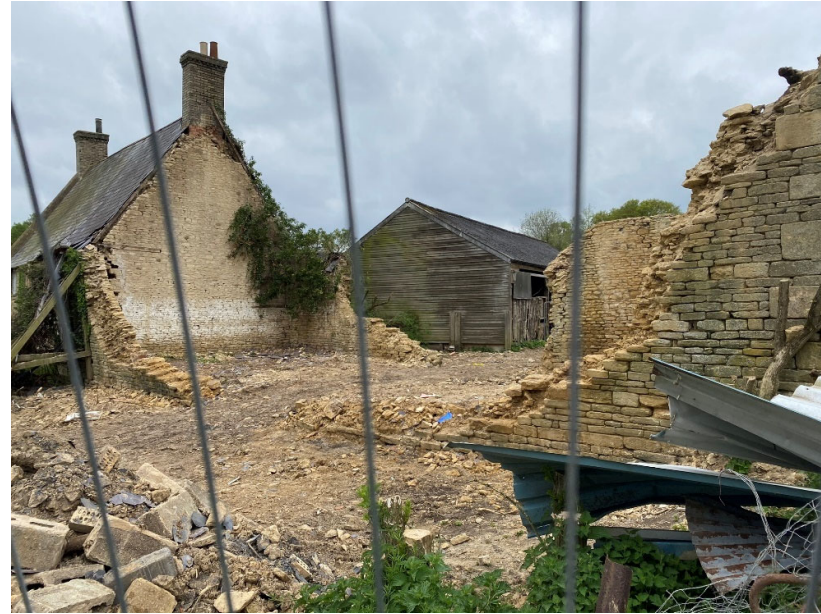
Cottage 2 end elevation and collapsed barn
