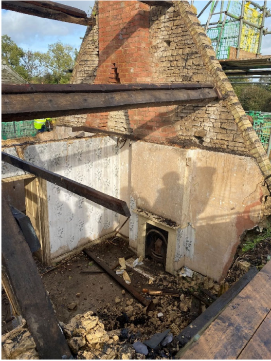
Cottage 2 removed section of roof and gable end
