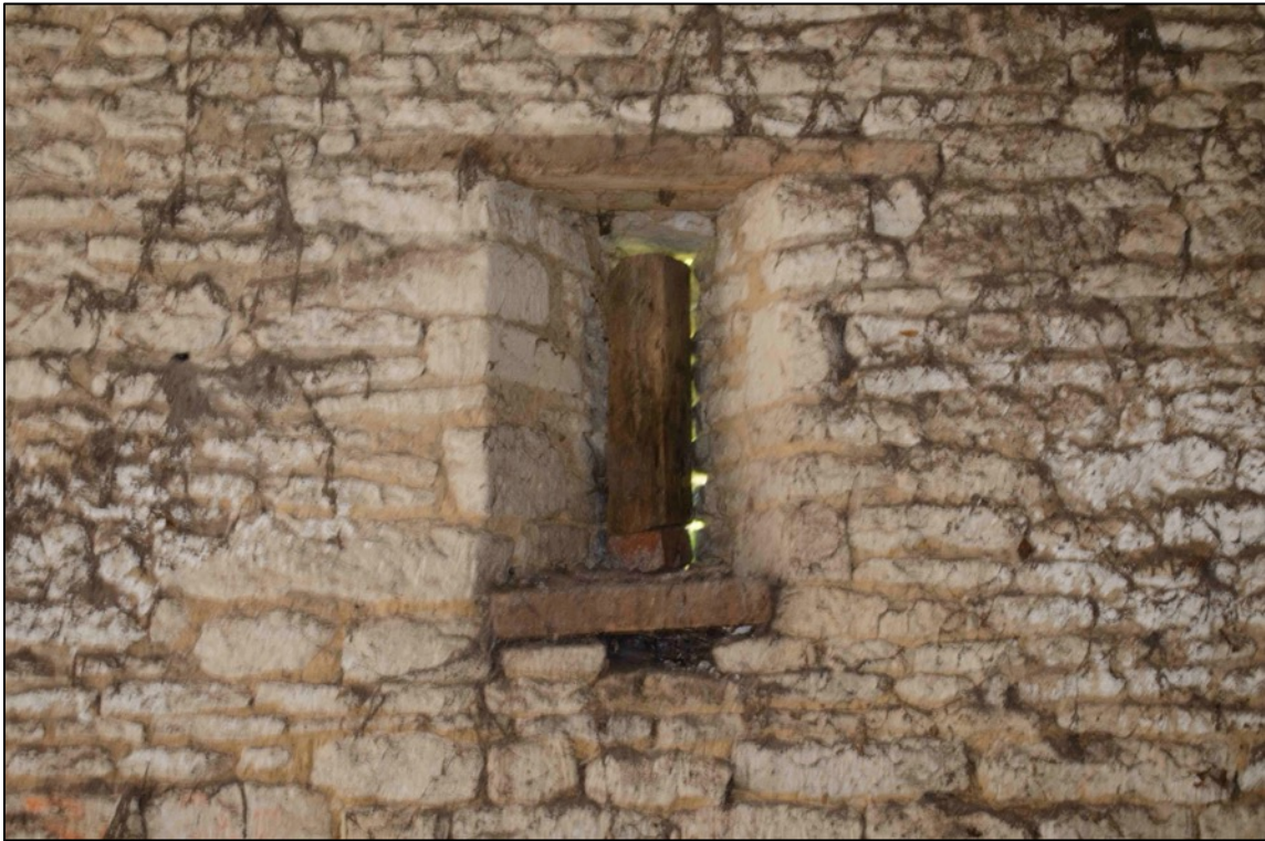
Appendix 2.41 Detail of blocked ventilation slot in south-east wall of room IG9, Barn I (2018)
