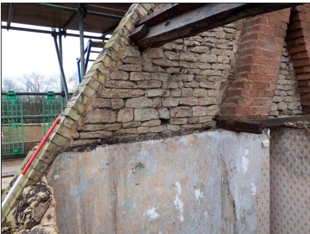
Appendix 2.32 View of roof of Cottage 1 , looking east, showing alterations to internal wall (2023)
