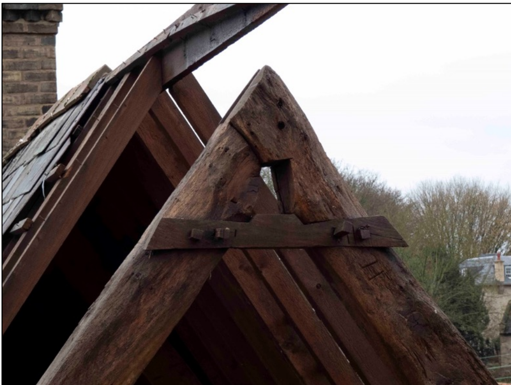
Appendix 2.36 Detail of truss above Cottage I showing joint at apex of principal rafters, looking south-east.
