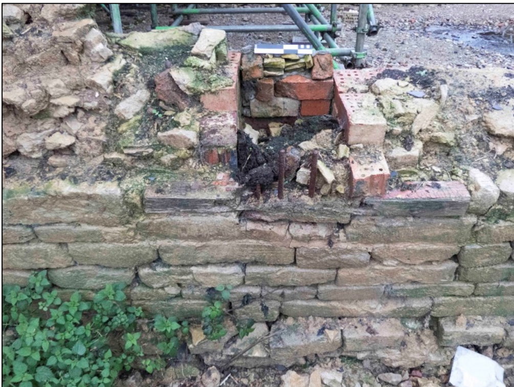
Appendix 2.40 Detail of inserted 20 th century brick feature in south-east elevation of Barn I (2023)
