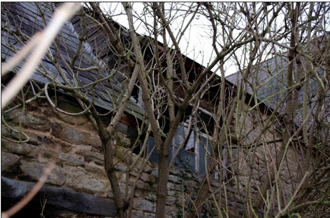
Appendix 2.48 Detail of window and change in roof pitch in south-west elevation of Barn 2, looking east (2018)
