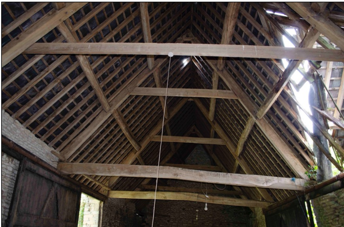
Appendix 2.46 Detail of roof structure of Barn I above room IG9, looking south-west.
