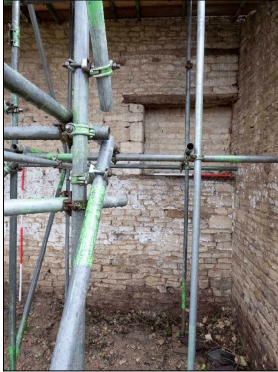
Appendix 2.45 Detail of blocking in south-west wall of room IG9 Barn I (2023)
