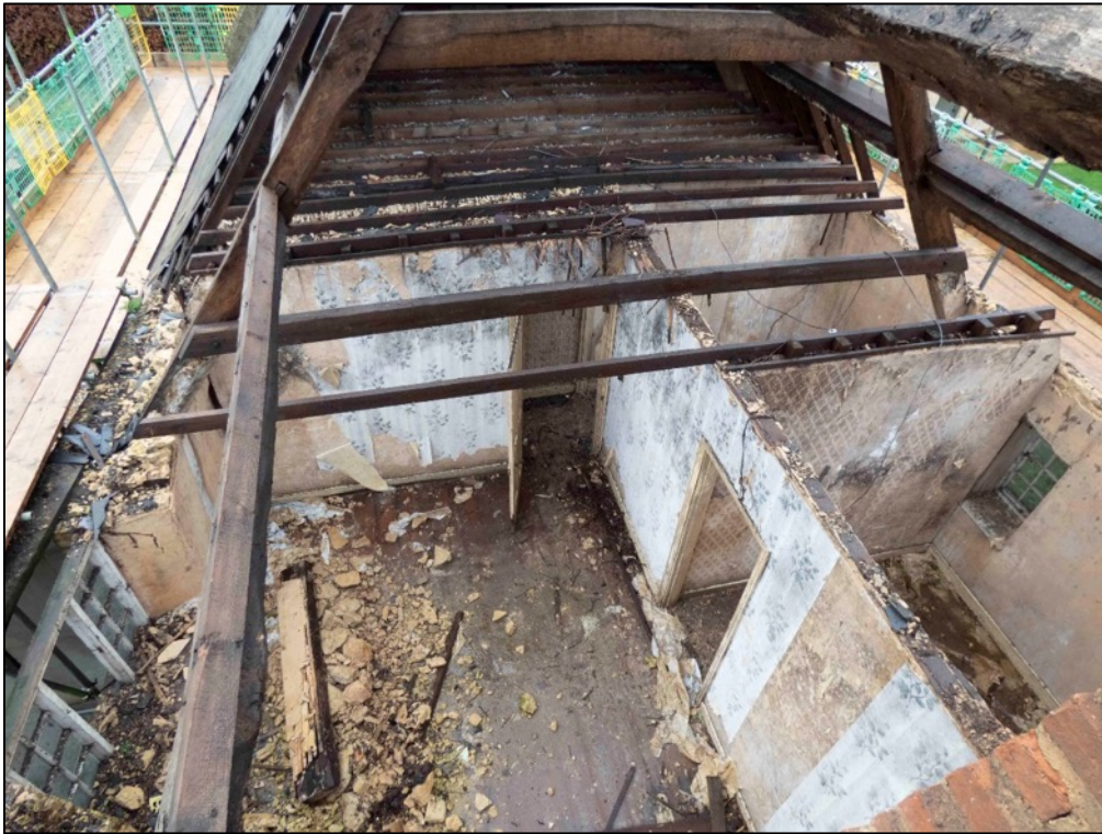
Appendix 2.33 View of roof of Cottage I , looking south-west down into rooms IG5-IG8
