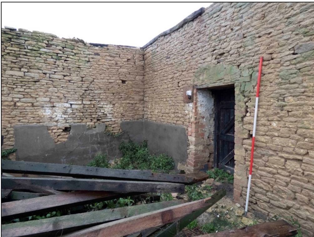
Appendix 2.42 Detail of door and concrete skim to wall in IG9, Barn I, looking north (2023)
