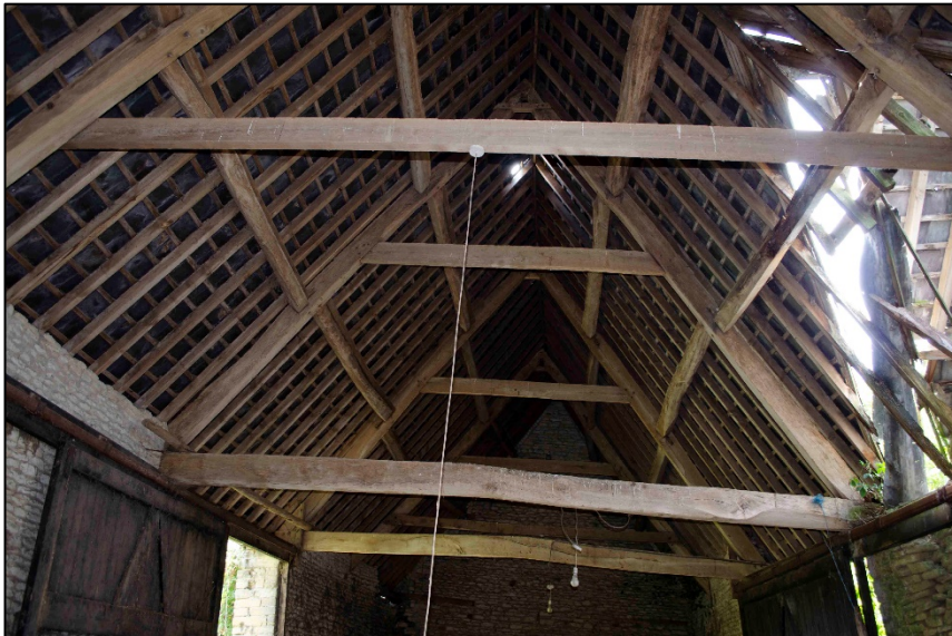
Appendix I.17: Detail of roof structure of the Barn above room IG9 , looking south-west
