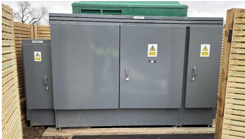
Figure 3: Feeder Pillar and COP metering box
