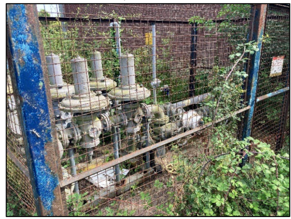
Plate 6. Gas installation cage on the northern perimeter of the Site.
