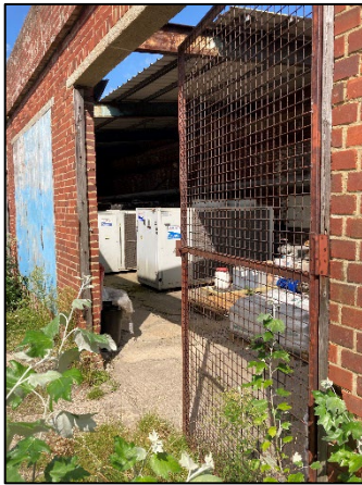
Plate 9. Cooling shed on western perimeter of Site.
