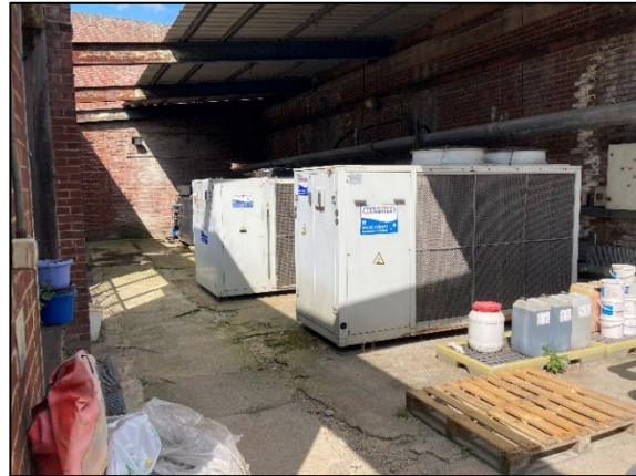
Plate 10. Small coolant tanks inside cooling shed.
