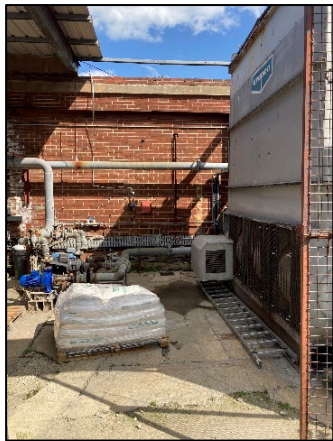
Plate 11. Large coolant tank inside cooling shed.
