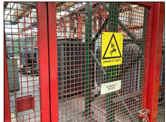
Plate 16. Electrical substation in centre of factory main shop.
