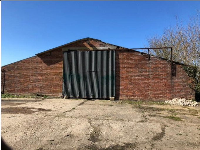
Photo 1 A view of the eastern elevation of the existing farm building, with hardstanding off the road access.
