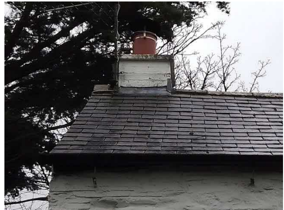
Photograph 4 – View of the lead seal around the chimney.
