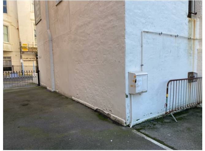
2 Existing gas meter and view towards carpark entrance off Paston Place
