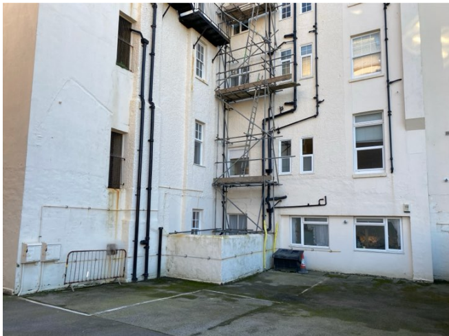
5 Rear elevations with additional gas meter, pipework and boiler flue to flat 16
