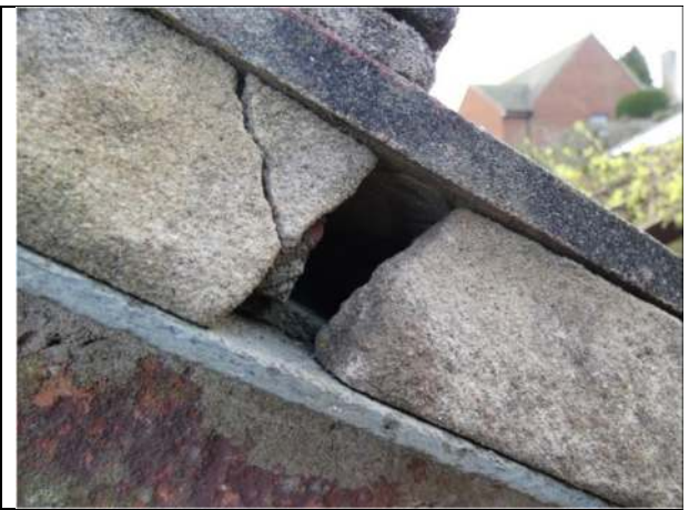
Photograph 16. Crack in the mortar along the northern edge of the garage roof
