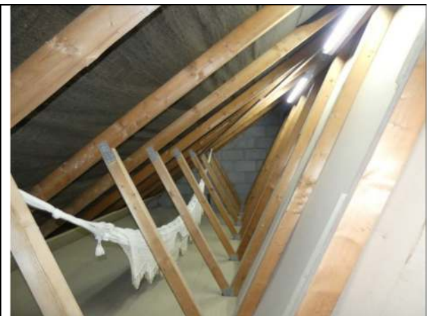
Photograph 18. Example of the void just outside the converted roof space in the garage
