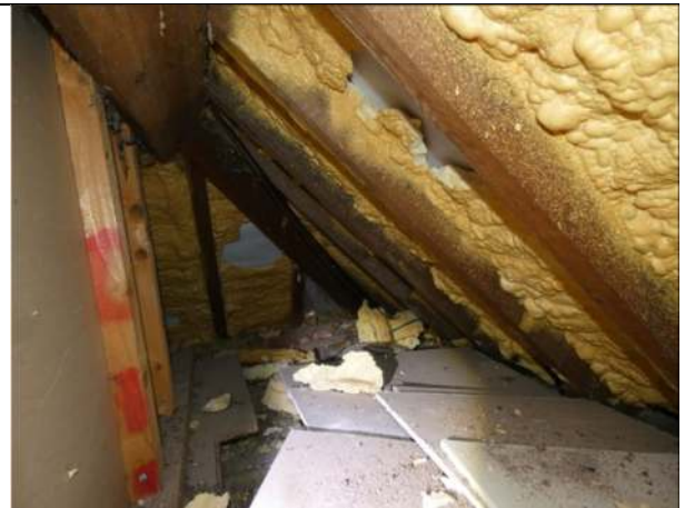
Photograph 10. Cavity along the edge of the roof void in the house (not expanding foam)
