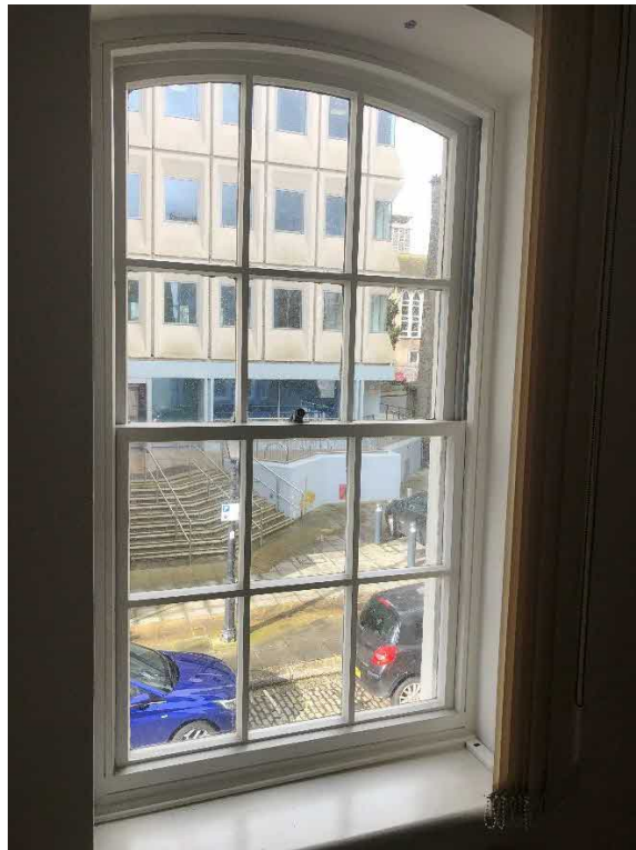
Typical sash type window of the property which is to be retained.
