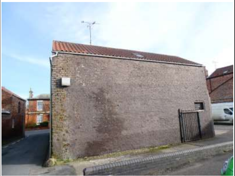
Western Boundary – Access Road to Rear Car Park at 47/48 Middle Street North
