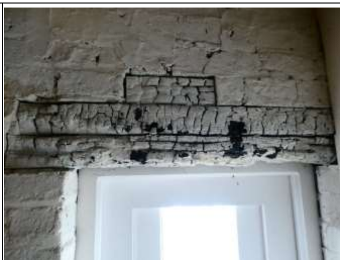
Charred Timbers Over Doorway
