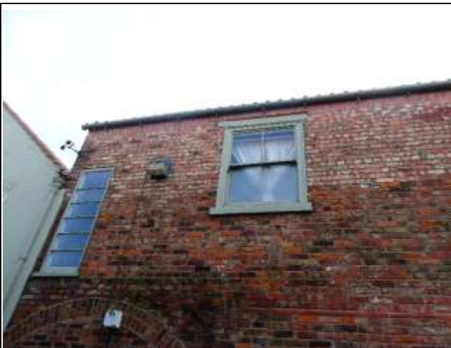
Stairwell Multi Pane Vertical Window and Timber Sash Window at the First Floor Front Bedroom
