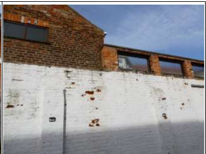
Section of Courtyard Walling on Top of the Protruding Section of the Elevation
